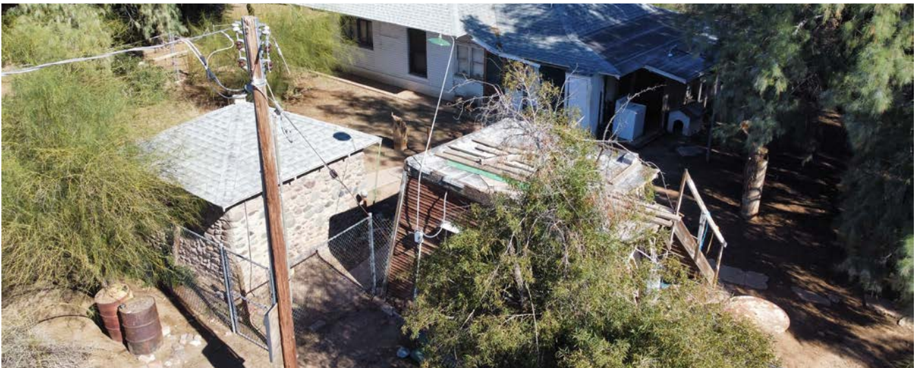
FIGURE EE: DETERIORATING STRUCTURES, HEATING OIL DRUMS, AND ELECTRICAL POLE
