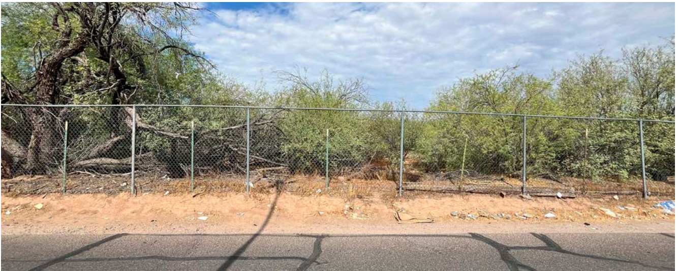
FIGURE CC: INADEQUATE AND DAMAGED FENCING
