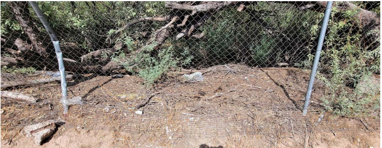
FIGURE Y: TAMPTERED CHAIN LINK FENCE
