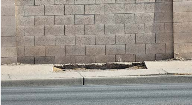
FIGURE D: DETERIORATING SIDEWALKS
