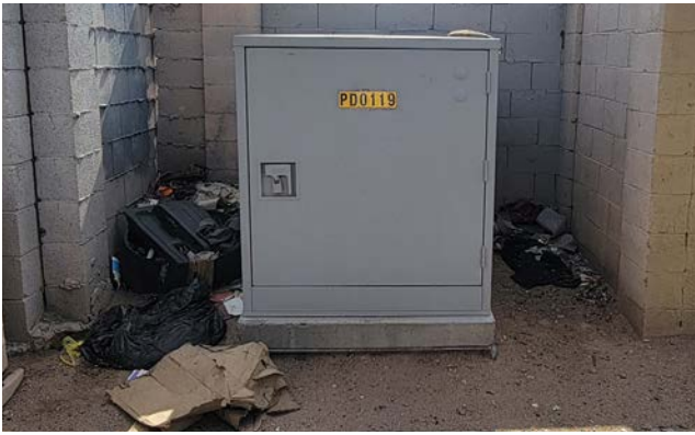
FIGURE R: ADJACENT ELECTRICAL BOX
