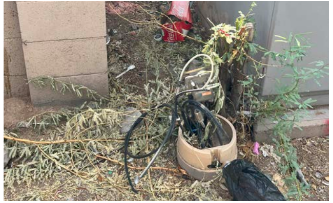
FIGURE O: EXPOSED ELECTRICAL
