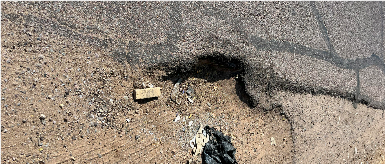
FIGURE Z: DETERIORATING PAVEMENT EDGE
