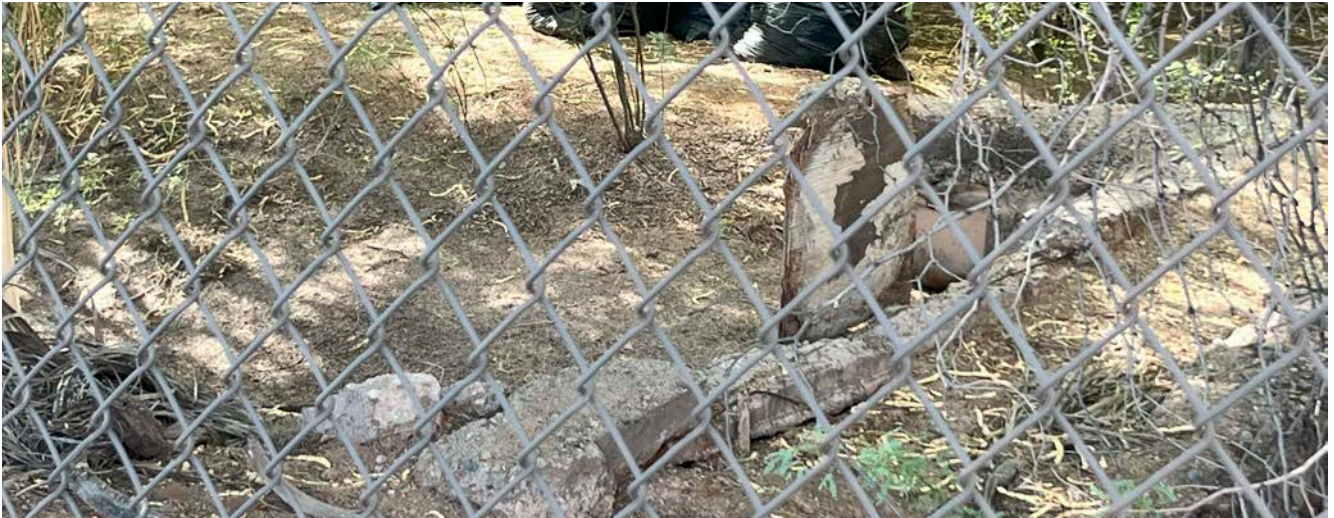
FIGURE AA: DETERIORATING CONCRETE IRRIGATION DITCH
