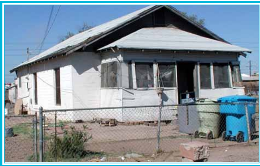
Figure 20 - Poor housing condition
