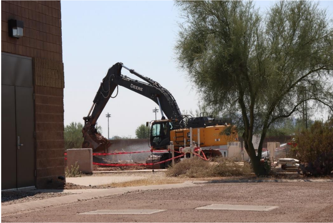
Demolition of old facilities taking place at the Cave Creek Water Reclamation Plant
