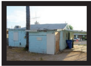
Dilapidated and unsafe homes
