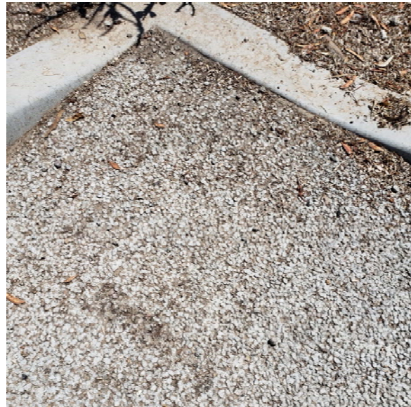
Sediment buildup at sump locations
