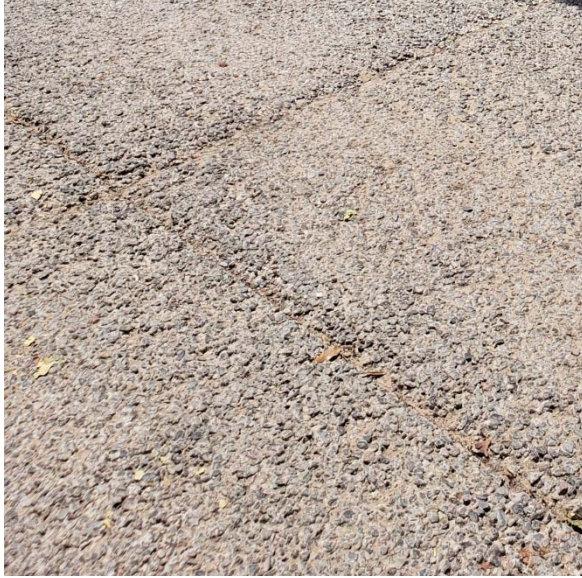
Sediment filling surface voids
