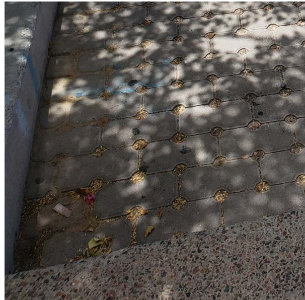
Debris on Pavers
