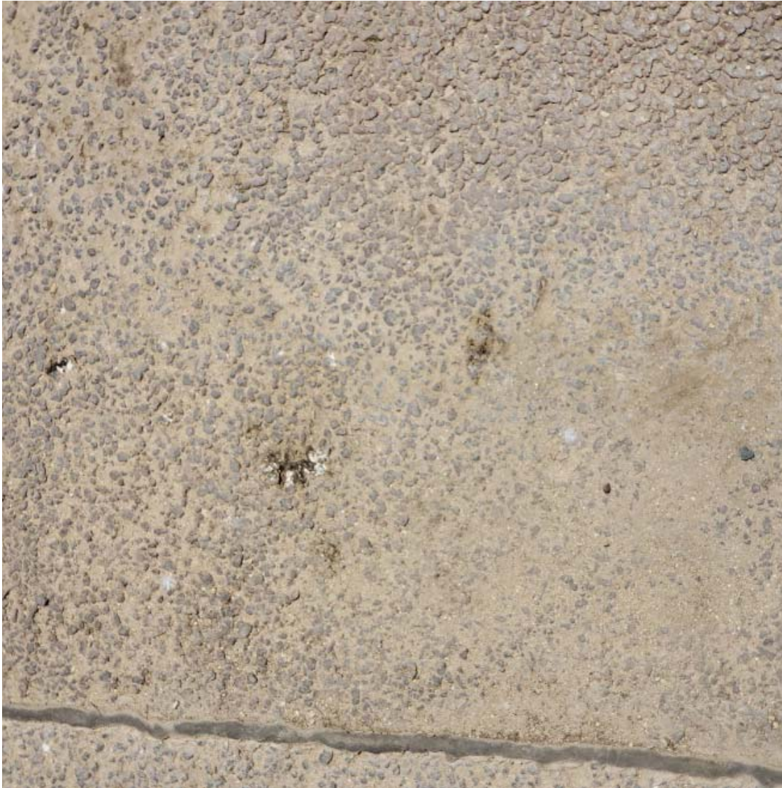
Pervious concrete full of sediment
