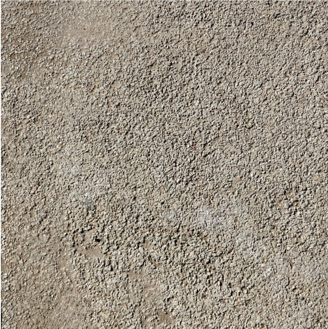
Sediment filling surface voids
