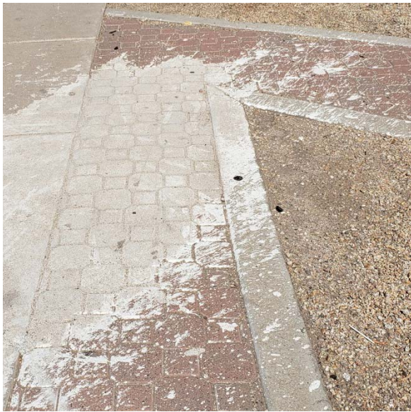
Paint spill over pavers
