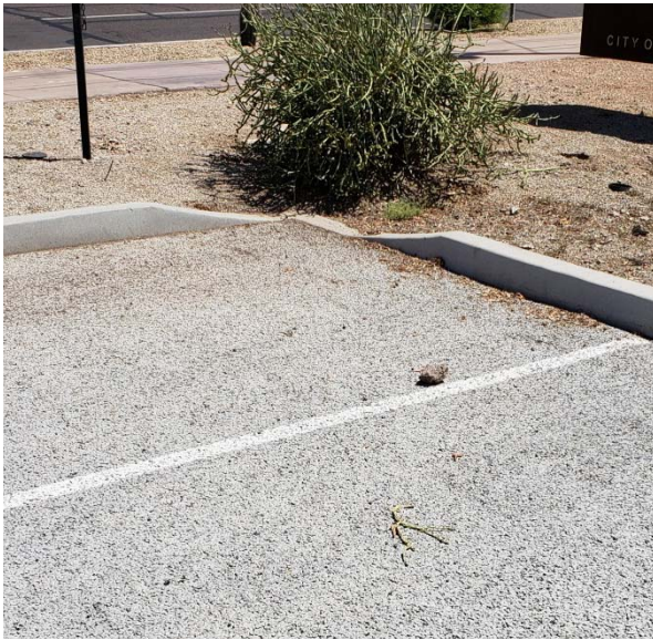
Debris buildup at sump locations
