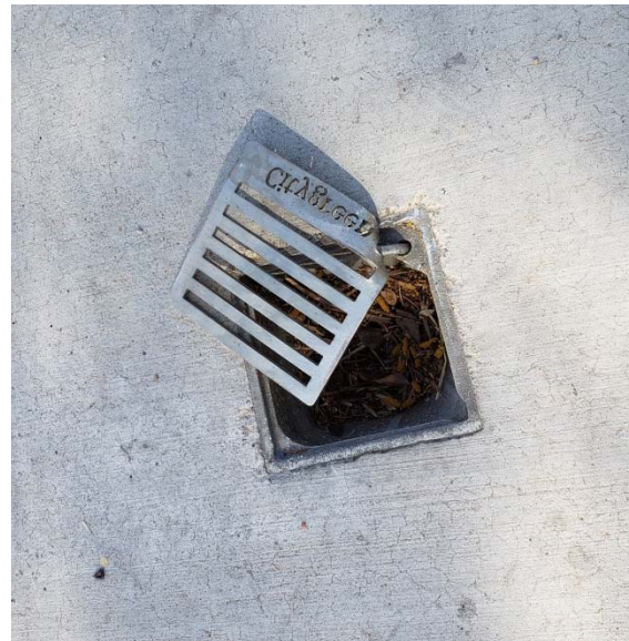
Clogged drain inlet
