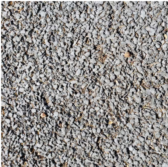
Pervious conc. partially clogged with debris
