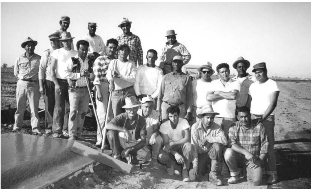
Invented at John F. Long, this sidewalk/rolled curb apparatus does the work of four men, averaging 600' feed of sidewalk/curb per hour. Long set the standards for infrastructure and sidewalks became part of all new subdivisions in the area. Photo courtesy of John F. Long Properties
