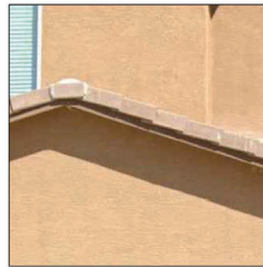
CONCRETE TILE AT RAKE
