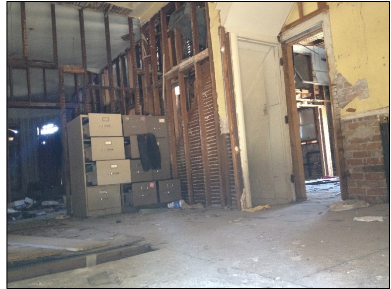
Photo 14. Interior view of house, looking through hole at southeast corner.
