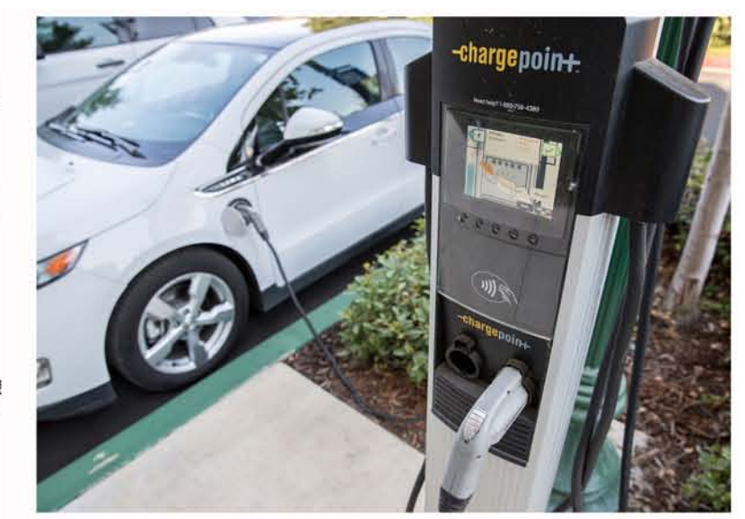
ELECTRIC VEHICLE CHARGING STATION
