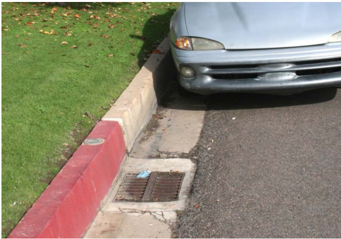
Existing tall old style curbs are a safety issue for pedestrians and can be damaging to vehicle doors and bumpers.
