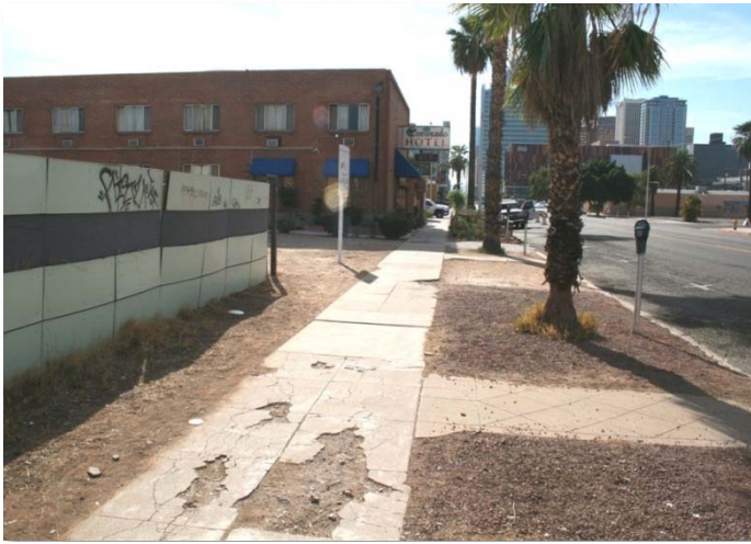
Aging sidewalk needs to be replaced in many areas.
